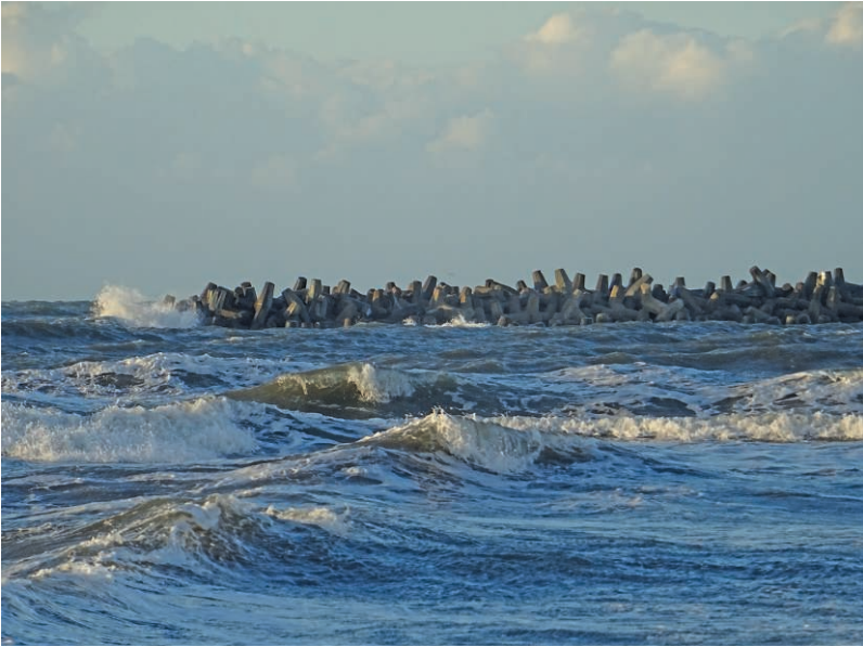
Figures 2a. Coastal defence structures: offshore breakwaters in Ras el-Bar. Source: F. Bonnefoi, March and April 2021.
