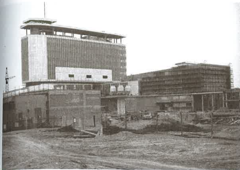
FIGURE 11.1 The CST staff tried to resist the occupation by keeping broadcasting at all costs. They were transmitting from a building under construction in Kavčí Hory (above), from transmitters Kojál and Cukrák, and from a military transmitter on Klet'. (Source: APF CT, 1968).
