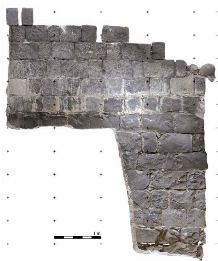
Fig. 19. The propylaeum. The eastern wall of the western tower. Photogrammetry based side view
