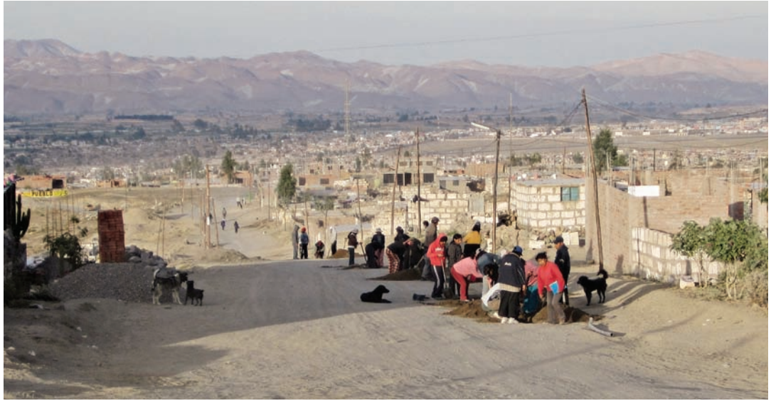
Settlers in a marginal neighbourhood fixing water infrastructure in a collective work session.
