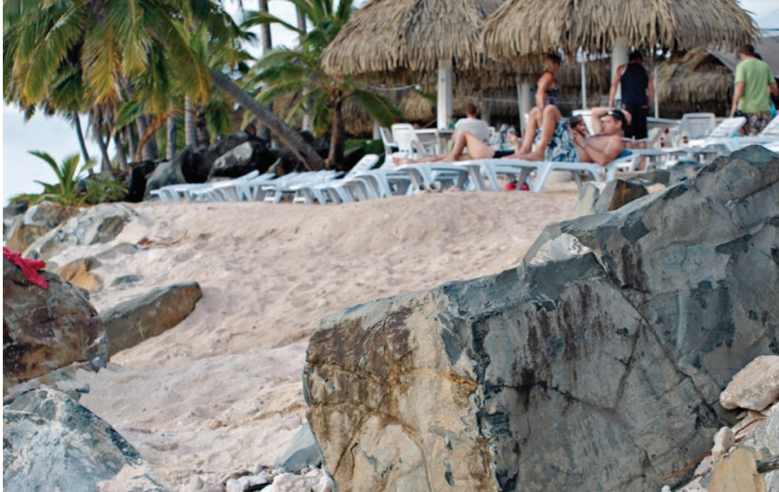
Blocks from a ruined coast protection due to storms and cyclones.
