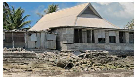
Even seawalls made from concrete cannot always protect houses against the ocean.
