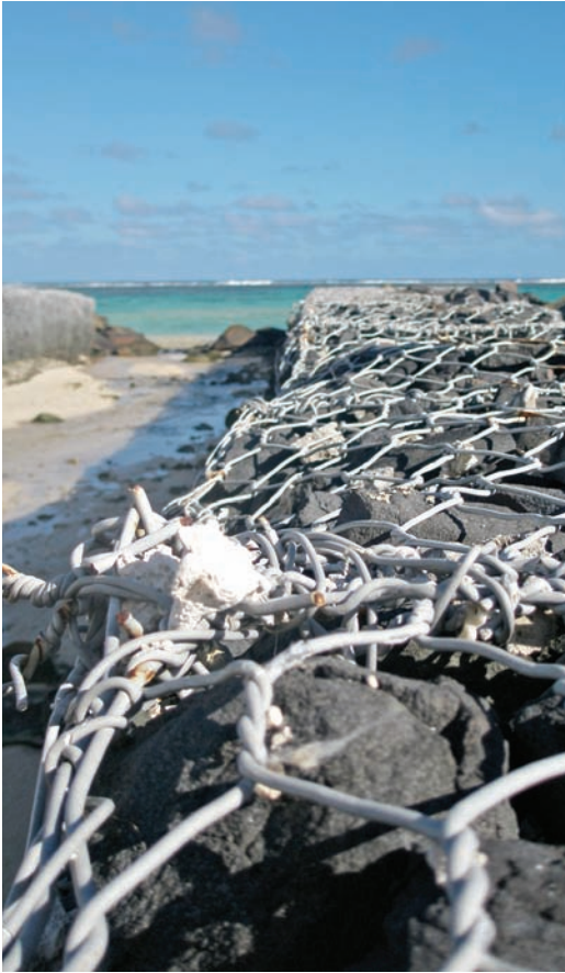
A newly made construction redirecting a stream that goes from the interior of Rarotonga to the lagoon.
