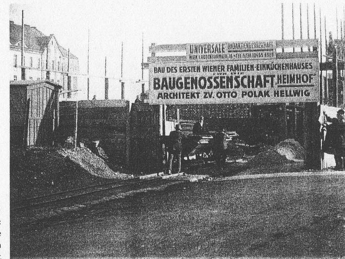
DAS EINKÜCHENHAUS (1923) Documentary footage: The construction of the residential complex in Vienna's 15 th district
