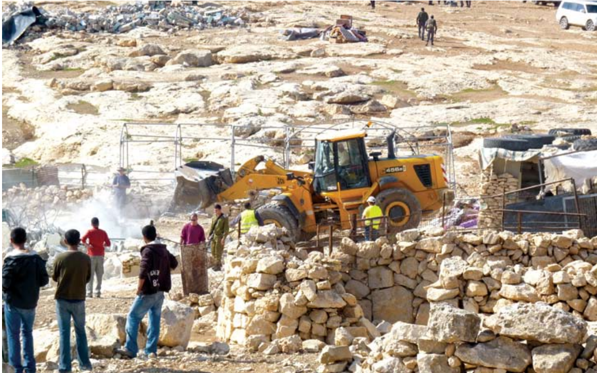
Demolitions at Khirbet al-Mufaqqarah in Firing Zone 918, South Hebron Hills. Photo: Nasser Nawaj'ah, B'Tselem, 24 November 2011.
